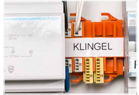
Example of a residential door bell application – carriers mounted on a DIN-35 rail
