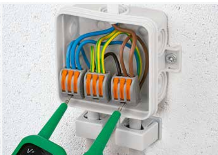
Testing the wired connectors.
